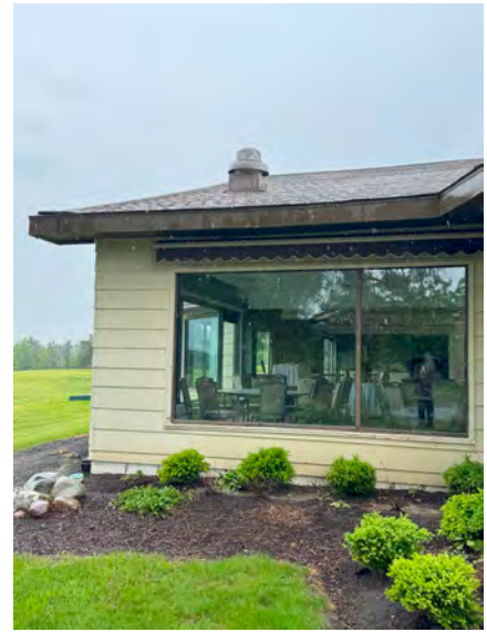
No Gutters at Slopped Roofs
