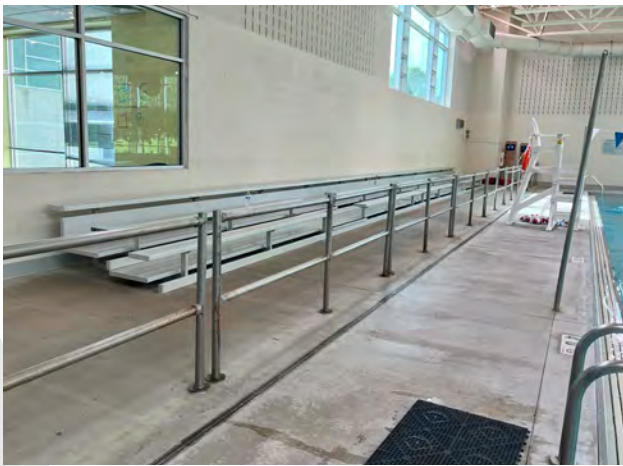
Splash Central - Rusted Railings
