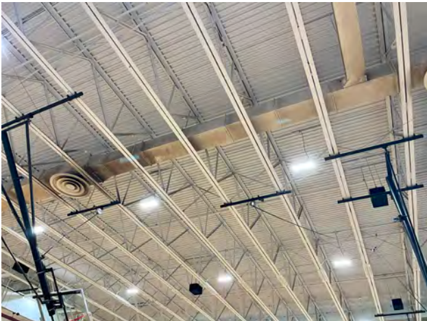
Gymnasium - Peeling Paint
