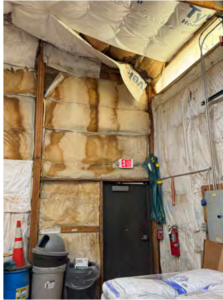
Golf - Damaged Interior Insulation
