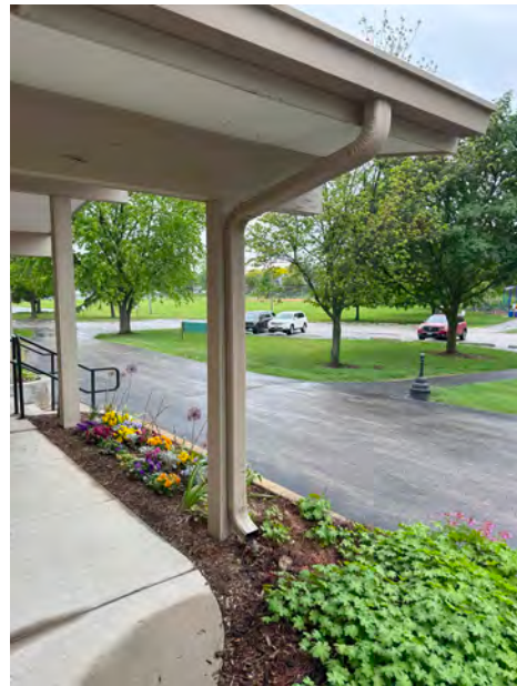
Downspout Discharges Next to Accessible Ramp and Pools on Sidewalk
