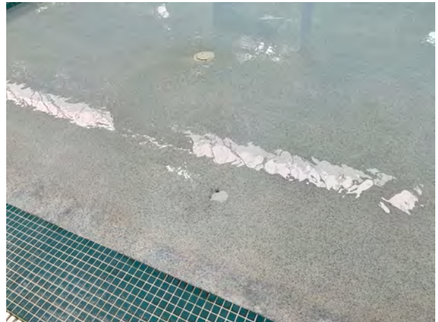
Splash Central - Peeling Pool Finish
