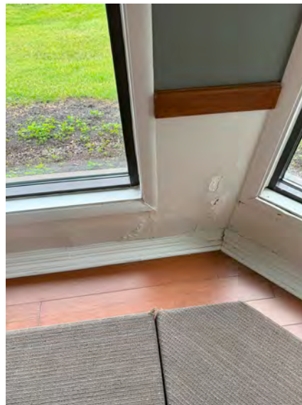
Water Damage on Interior Wall
