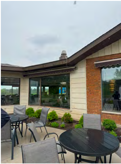
No Gutters at Slopped Roofs
