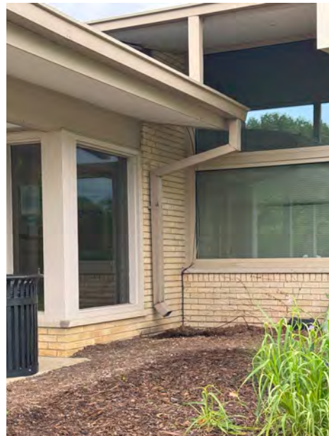
Downspout Discharges Next to Building Foundation
