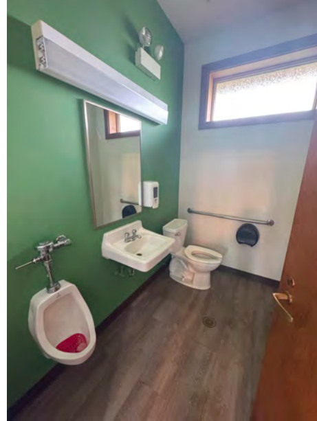
Toilet Rooms - ADA Compliance
