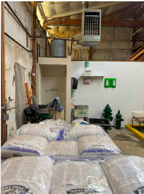
Golf - Non Compliance of Shower and Sink Plumbing Vent
