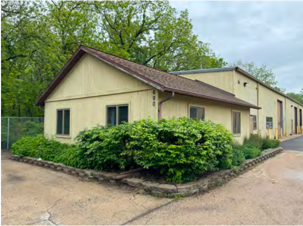
Exterior in Poor Condition
