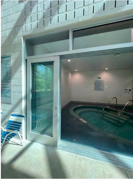
Splash Central - Broken Sliding Spa Door
