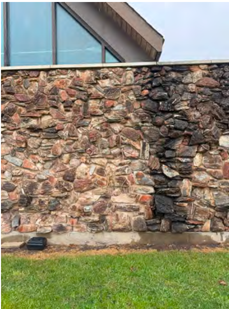
Water Staining on Stone from Rain
