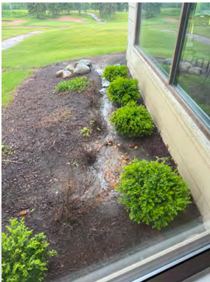
Water Ponding Near Foundation Due to Lack of Gutters
